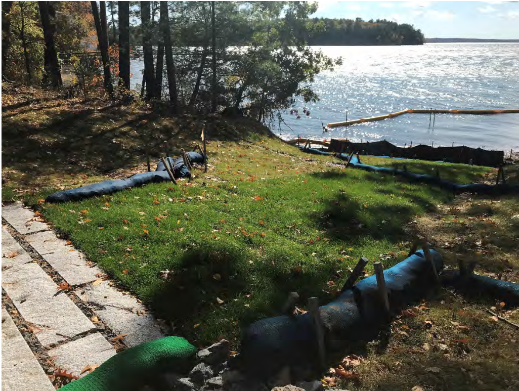
Fig 7: Slope below the manhole at Gundalow Landing/east side of the bay. Viewing south. (10-17-20)
