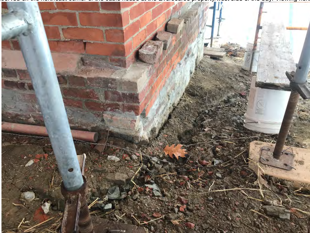
Fig 4: Rill observed on the southwest corner of the cable house at the Eversource property/west side of the bay. Viewing east. (10-17-20)
