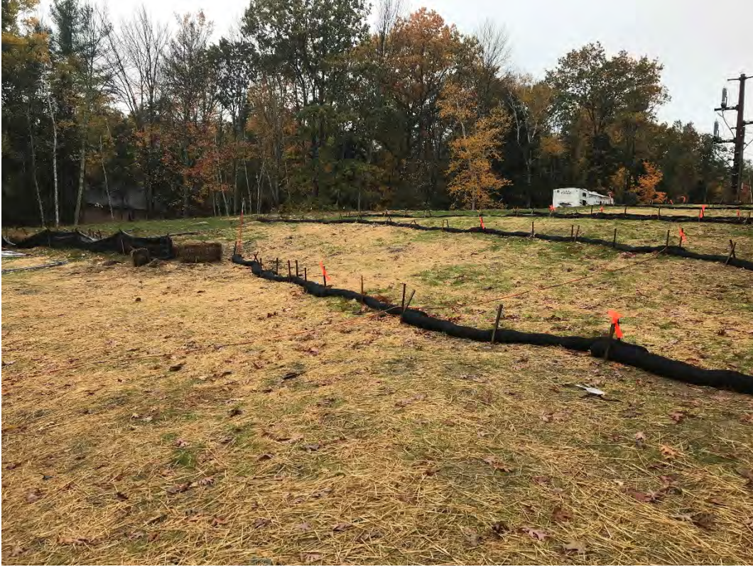
Fig 1: Slope above the cable house at the Eversource property/west side of the bay. Viewing southwest. (10-17-20)
