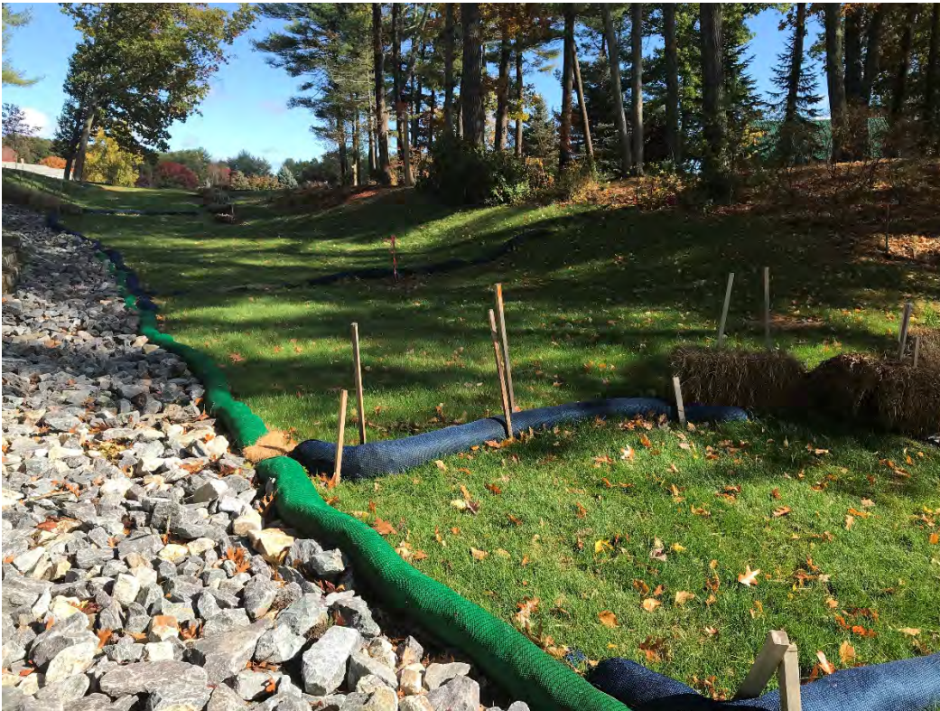
Fig 6: Slope above below the manhole at Gundalow Landing/east side of the bay. Viewing east. (10-17-20)
