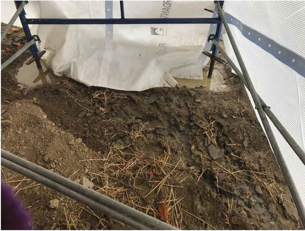
Fig 3: Rill observed off the northeast corner of the cable house at the Eversource property/west side of the bay. Viewing north. (10-17-20)
