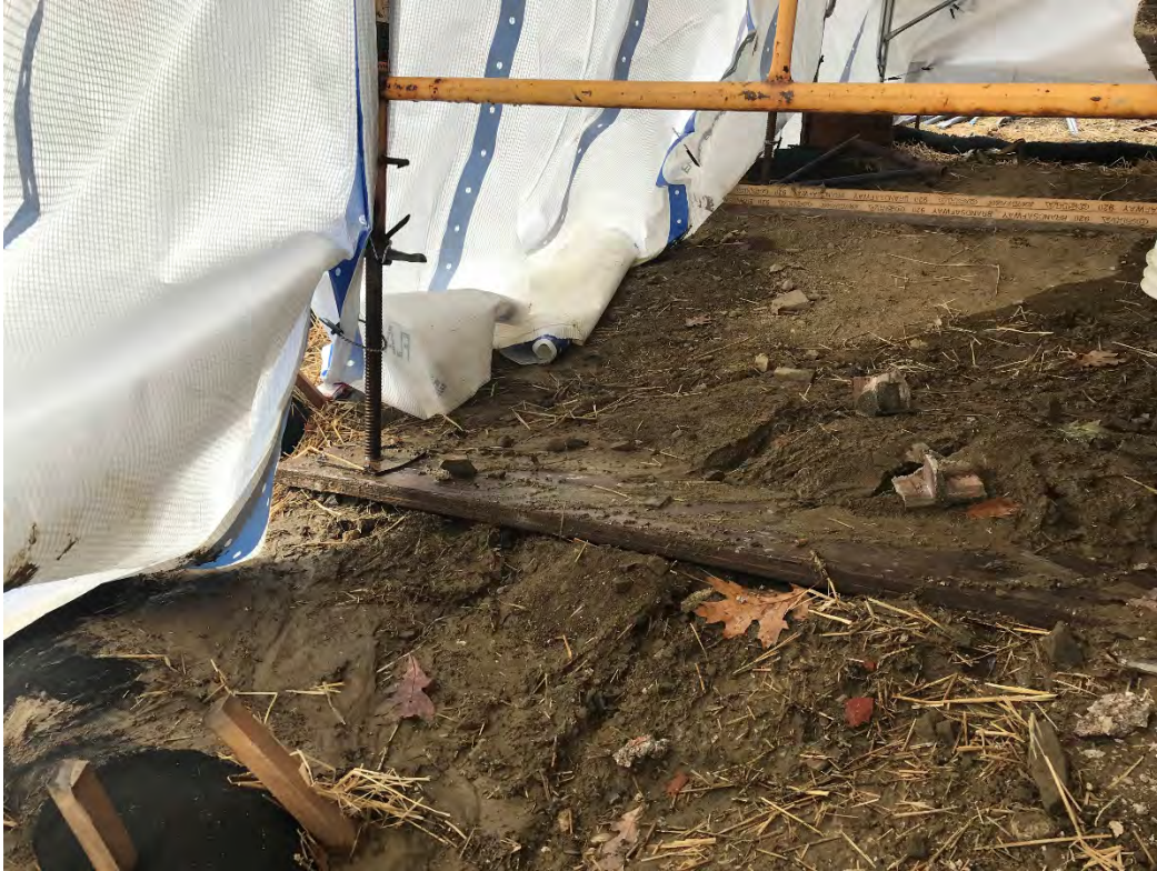
Fig 5. Rills observed off the southeast corner of the cable house at the Eversource property/west side of the bay. Viewing southwest. (10-17-20)
